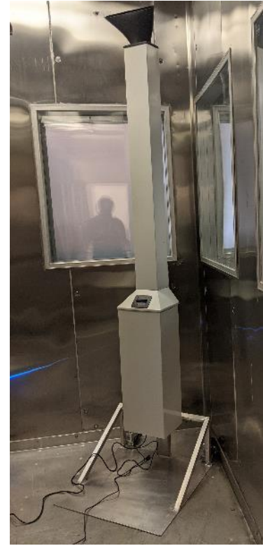
Figure 2. Location of uvcPhyzx Device Inside the DMTC.
